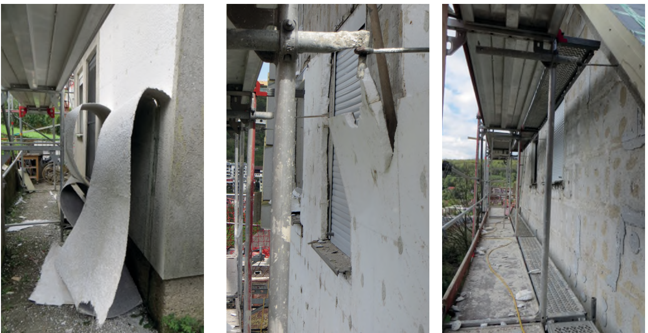
Figure 16 Left: selective dismantling of the rendering system creates a clean insulation surface. Middle: removal of the insulation layer from the wall. Right: stripping of existing ETICS leaves already a relatively clean wall (residuals of adhesive mortar visible). ©Ralf Pasker
